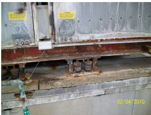
COOLING TOWER BASE – EXTENSIVE CORROSIVE DAMAGE
