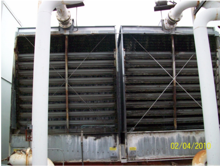
EXISTING BUILDING 2 COOLING TOWER
