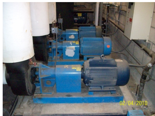
EXISTING CHILLED WATER PUMPS
