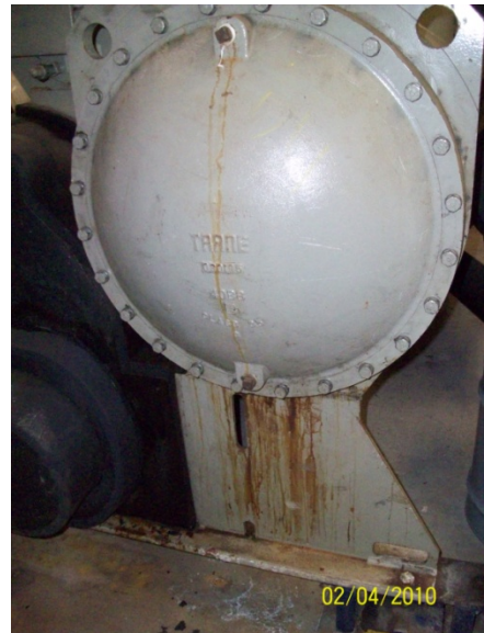
CHILLER - 2 - SIGNS OF LEAKAGE
