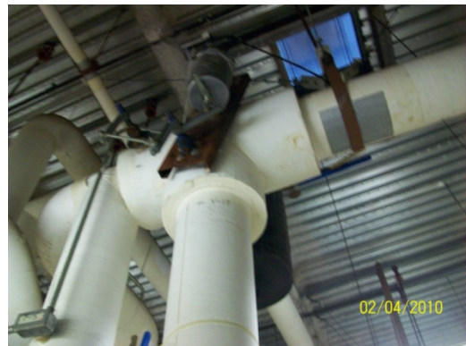
EXISTING PNEUMATIC CONTROLS
