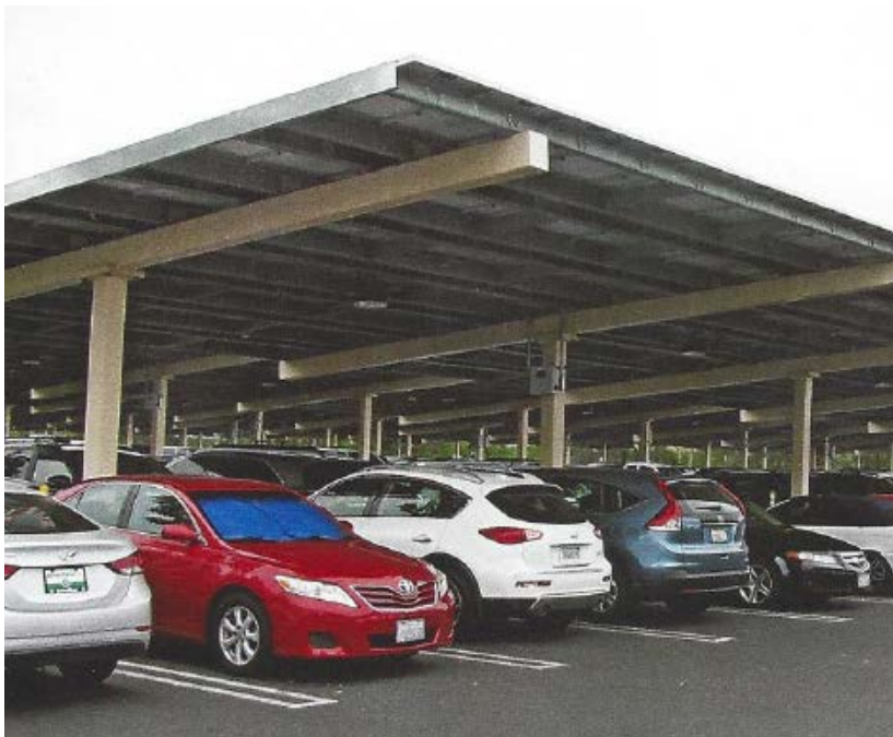
Exhibit 6.1: Solar Carport at Kaiser Permanente Hospital, Irvine
